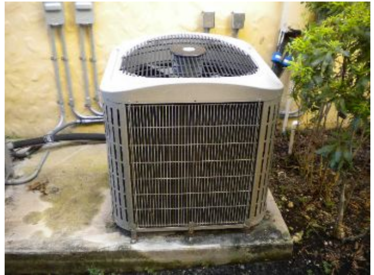
The air conditioner did not operate properly. Recommend HVAC contractor evaluate the system.
