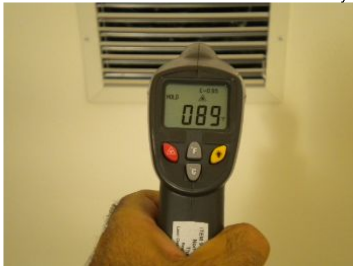
The typical temperature differential split between supply and return air in an air conditioner of this type is 14 - 22 degrees F. This system achieved an unacceptable differential temperature of 0 degrees F.
