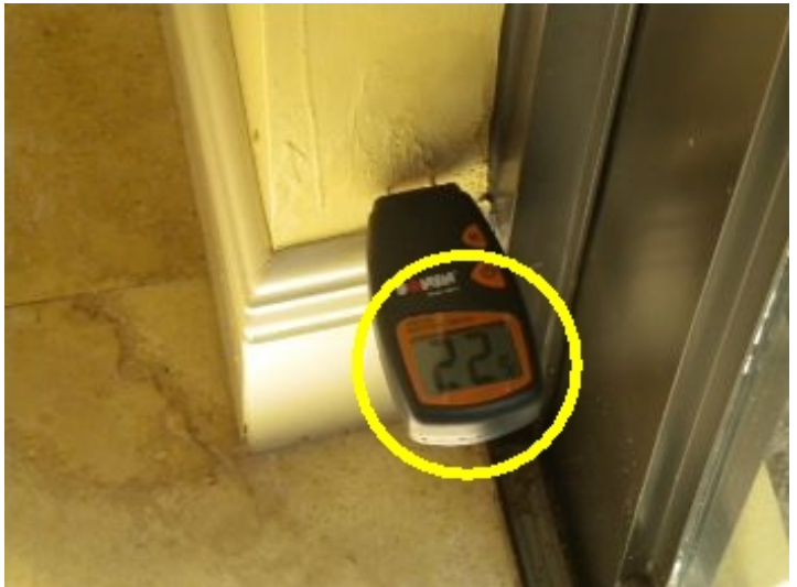
There is evidence of moisture entering structure at the bottom of the stairwell and inside the closet under the stairwell. Moisture readings were taken and exceed the acceptable level.
