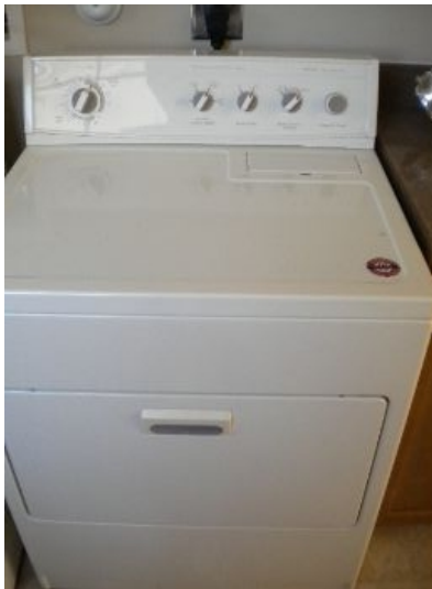
Dryer vent not connected
