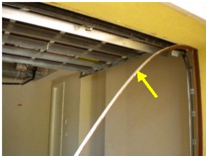
Garage Vehicle door trim is damaged.
