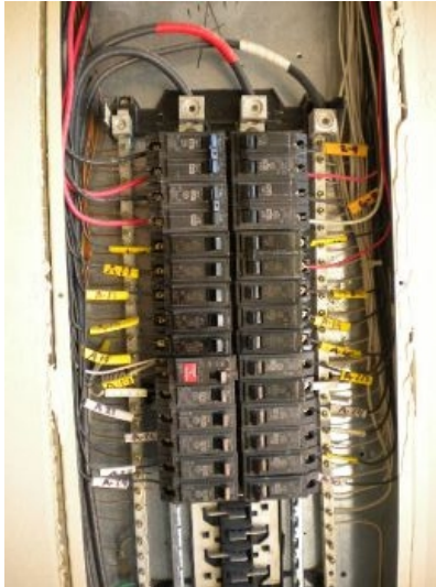
Electrical Electrical Panel
