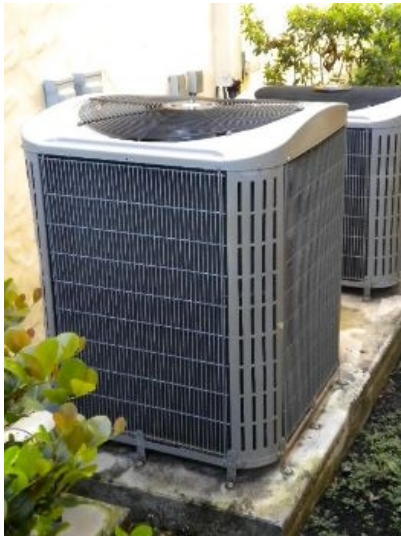
The air conditioner did not operate properly. Recommend HVAC contractor evaluate the system.
