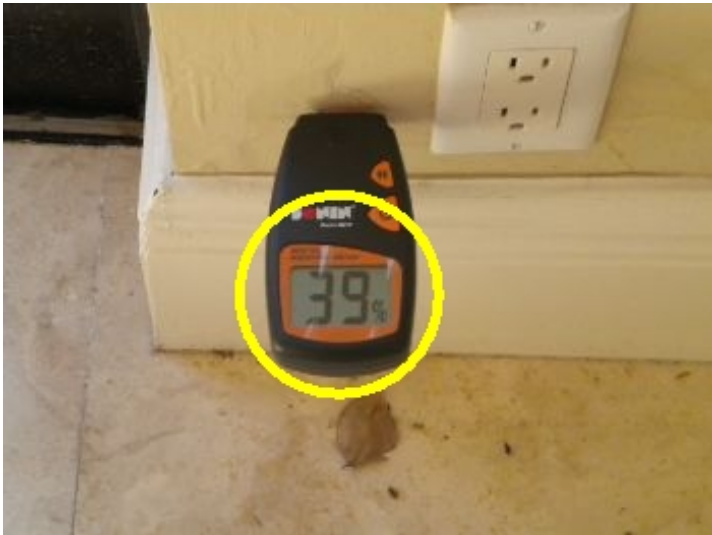
There is evidence of moisture entering structure at the bottom of the stairwell and inside the closet under the stairwell. Moisture readings were taken and exceed the acceptable level.
