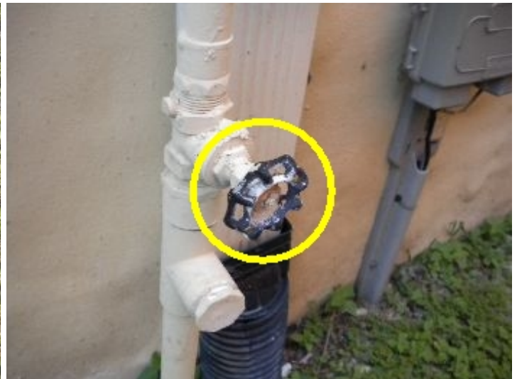
Water main located on East side
