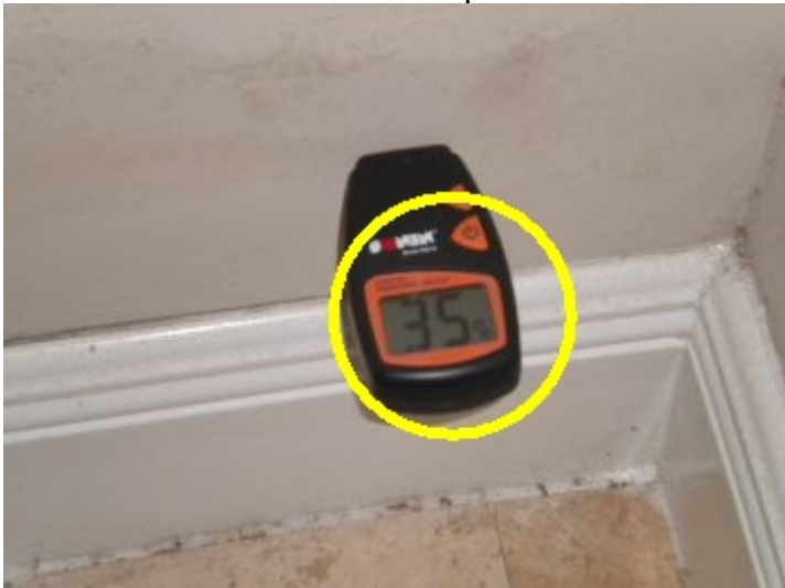
There is evidence of moisture entering structure at the bottom of the stairwell and inside the closet under the stairwell. Moisture readings were taken and exceed the acceptable level.
