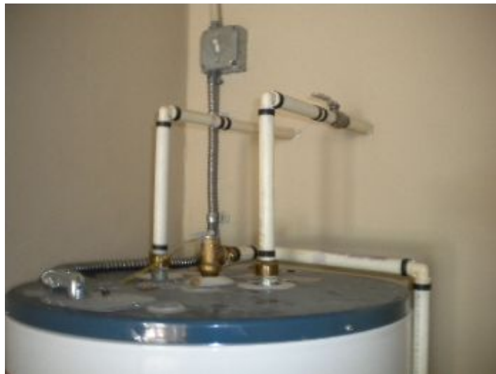
Water Heater Plumbing
