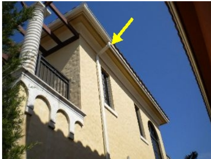
Partial gutters - Full installation recommended to keep water away from structure. Water can weaken the foundation.
