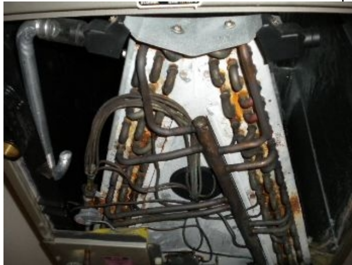
There is discoloration of coils due to the presence of defective drywall (Chinese drywall).
