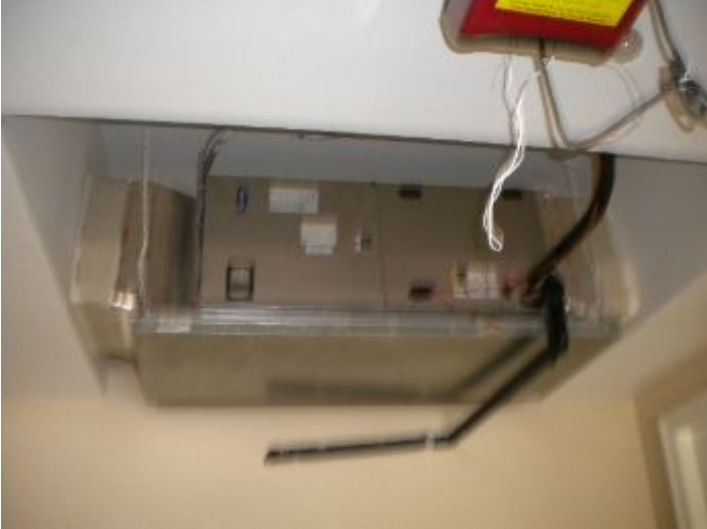
Units did not operate properly at time of inspection.
