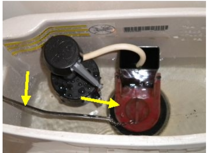
Mechanism in tank sticking, requires adjustment for proper flushing.
