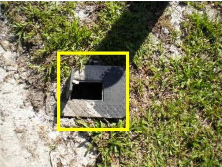
City water main
