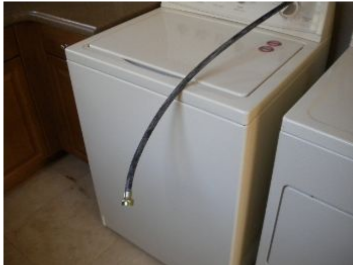
Unit was not hooked up to water supply at time of inspection.
