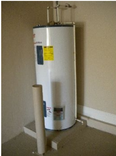
Water Heater Water Heater Condition
