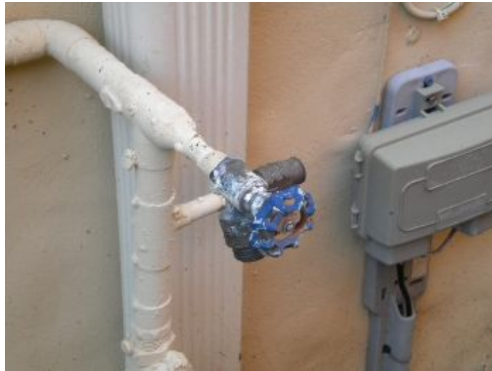
Grounds Exterior Faucet Condition
