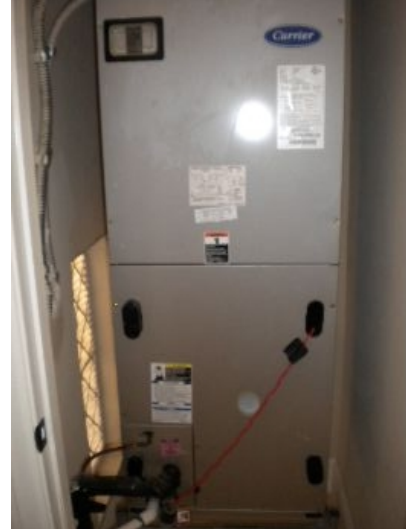
Units did not operate properly at time of inspection.
